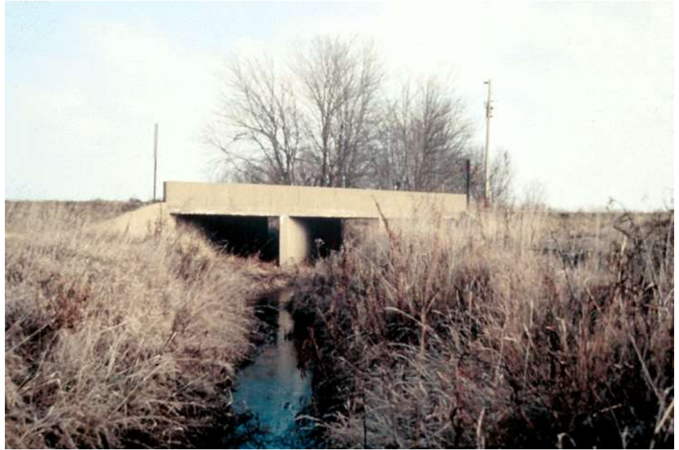
Figure 13.2.9 Vegetation Constricting the Waterway
