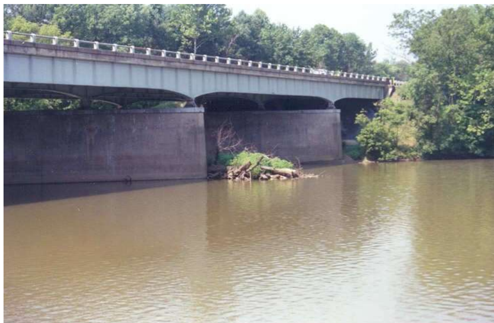
Figure 13.3.11 Buildup of Debris At Pier
