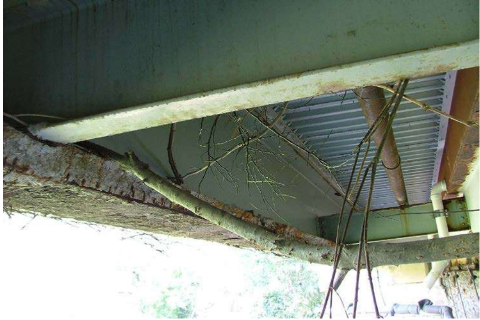
Figure 13.2.38 Drift Lodged in a Superstructure
