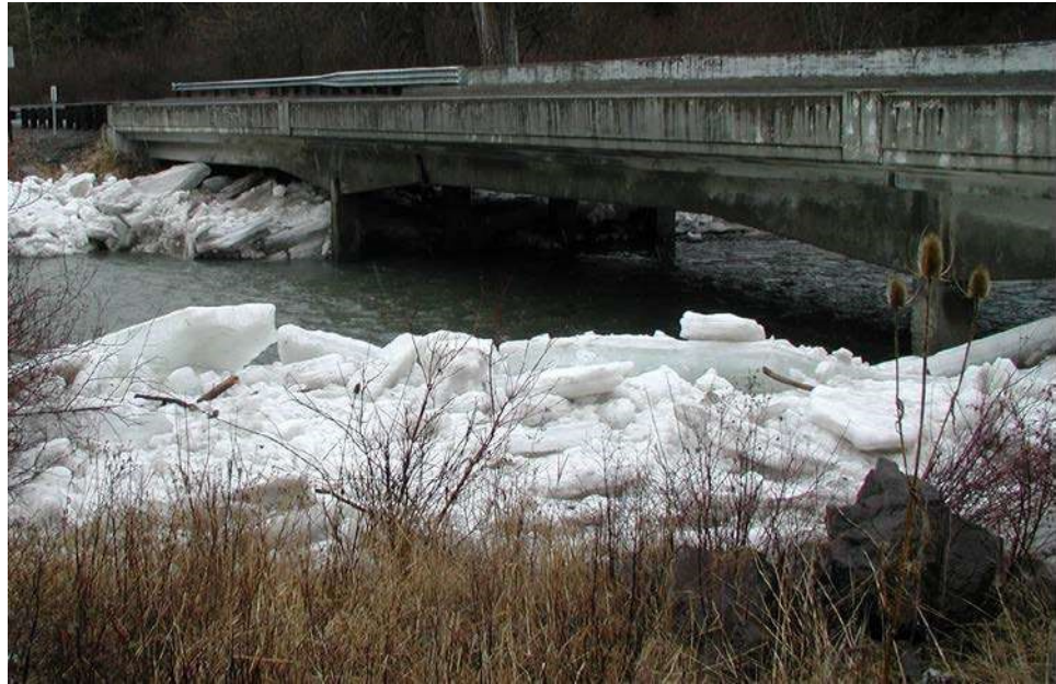
Figure 13.2.11 Ice in Stream Resulting in Possible Contraction Scour
