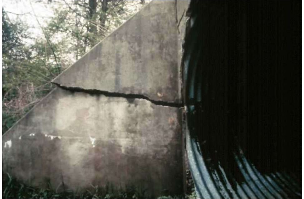
Figure 14.1.26 Cracking of Culvert End Treatment Due to Foundation Settlement
