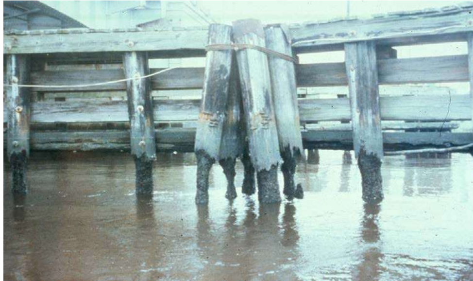
Figure 13.3.21 Damaged Protective System
