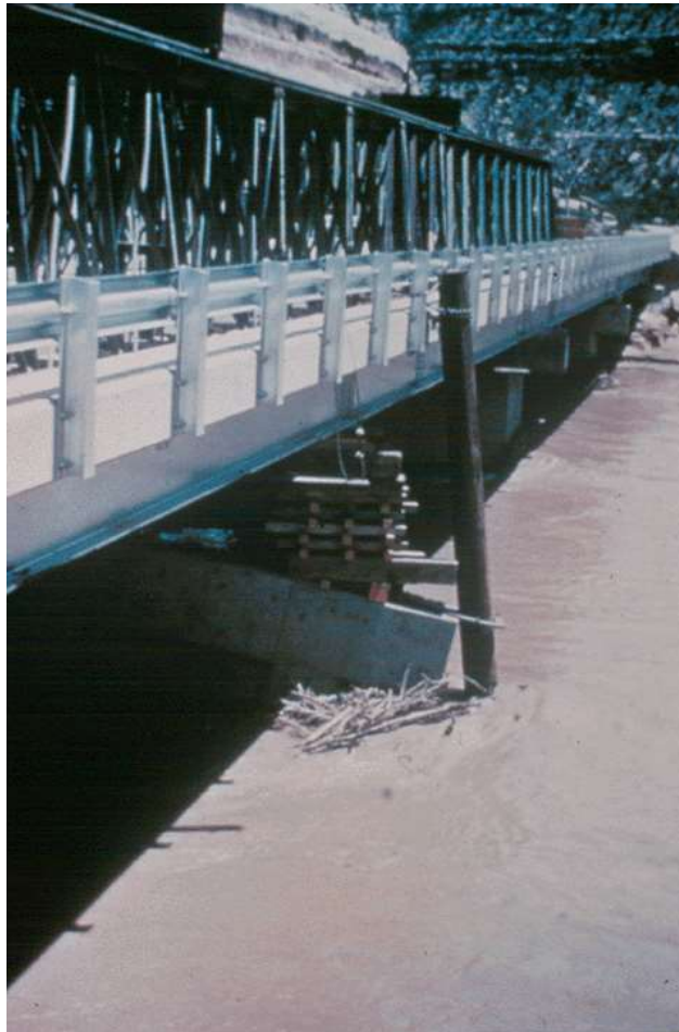
Figure 13.2.27 Pier Settlement due to Undermining
