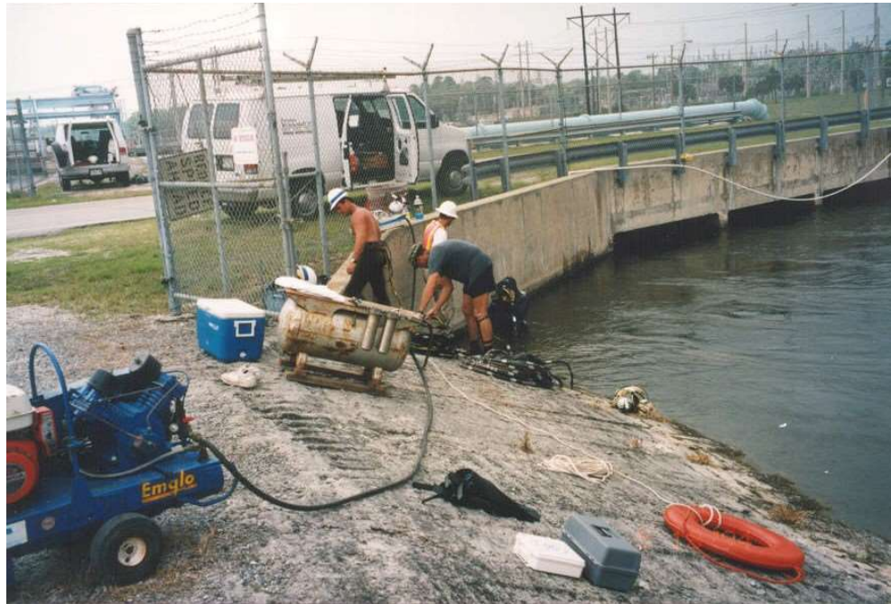
Figure 13.3.38 Surface-Supplied Air Equipment, Including Air Compressor, Volume Tank With Air Filters, and Umbilical Hoses
