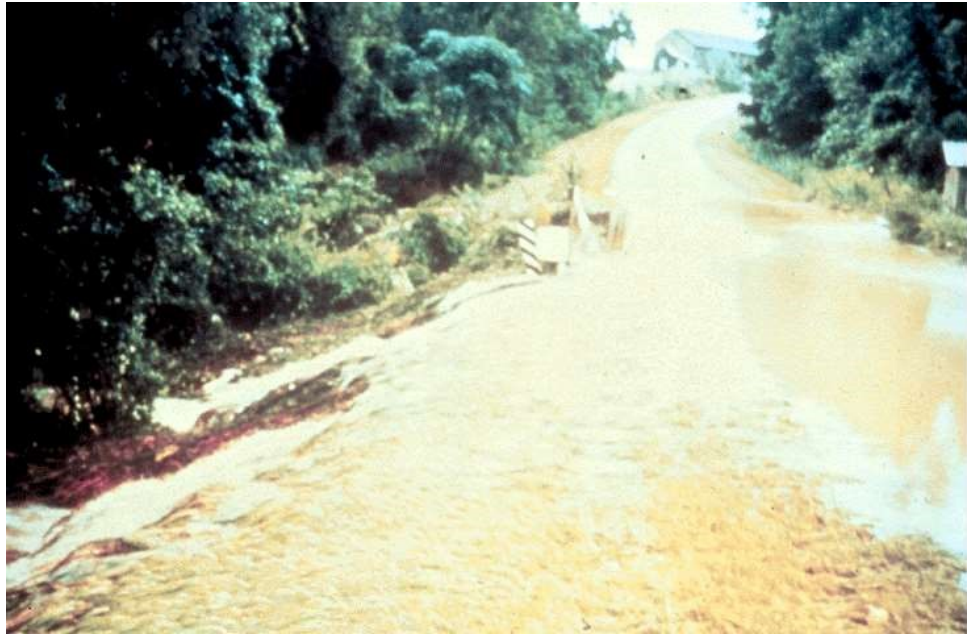
Figure 13.2.63 (Exhibit 63) Culvert Failure Due to Overtopping
