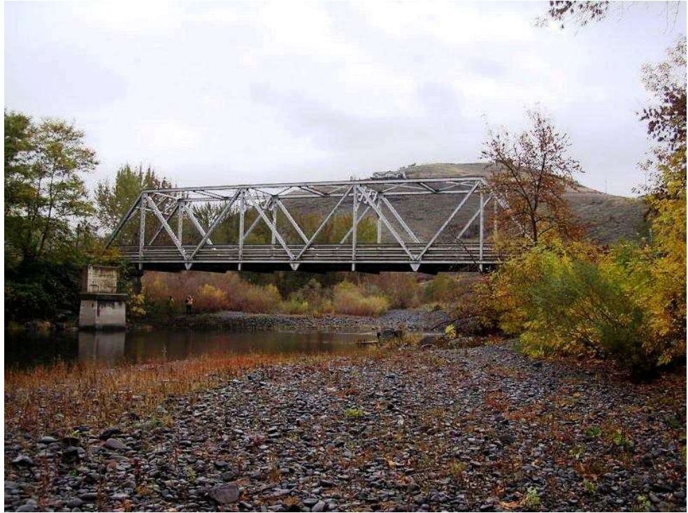
Figure 13.2.56 Stream Alignment Not Parallel with Abutments
