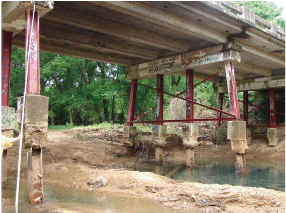
Figure 13.2.41 Severe Streambed Degradation Evident at Low Water
