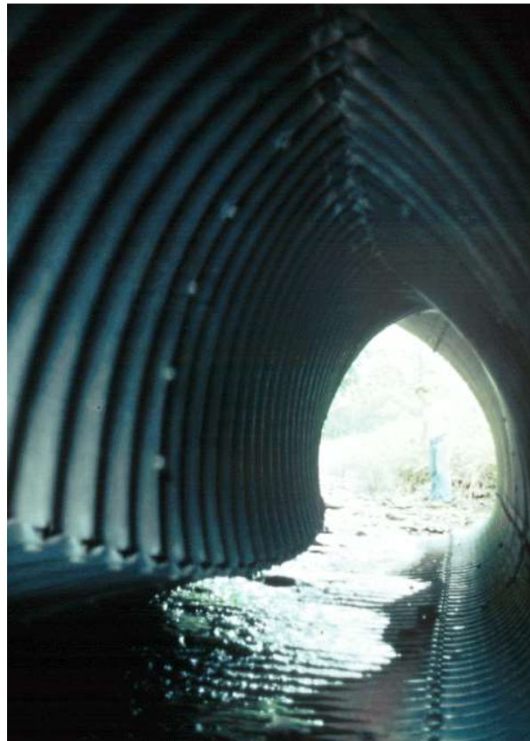
Figure 14.1.25 Bending or Shear Failure
