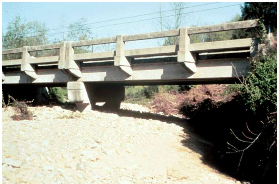
Figure 13.2.10 Sediment Deposits Within the Waterway Opening
