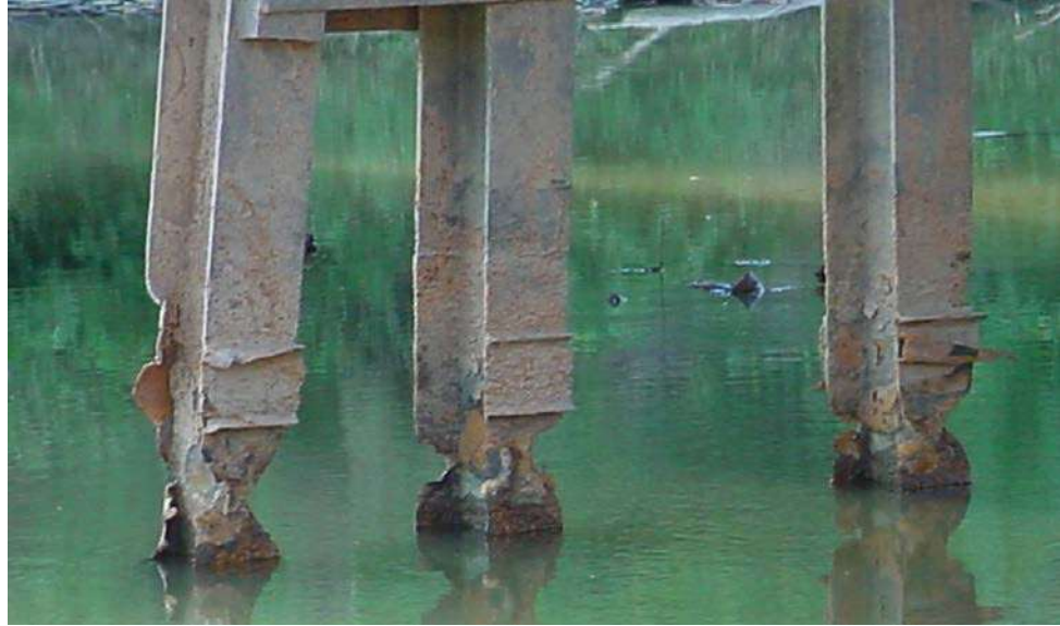
Figure 13.3.25 Deteriorated Steel Piles at Splash Zone
