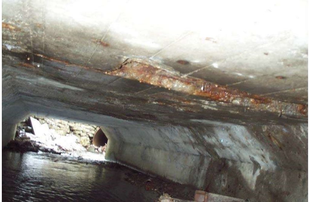
Figure 14.2.17 Spalls and Delaminations on Top Slab of Concrete Box Culvert
