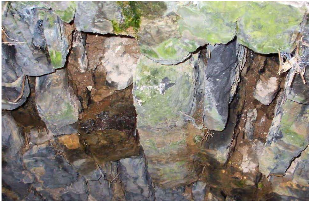
Figure 14.2.18 Missing Stones in Masonry Culvert
