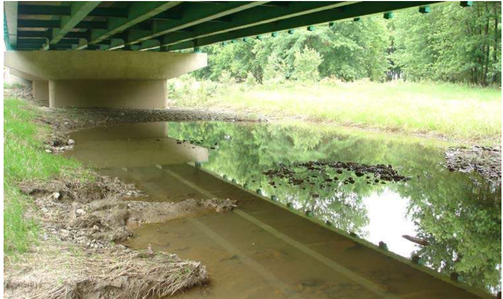
Figure 13.2.7 Contraction Scour Photograph
