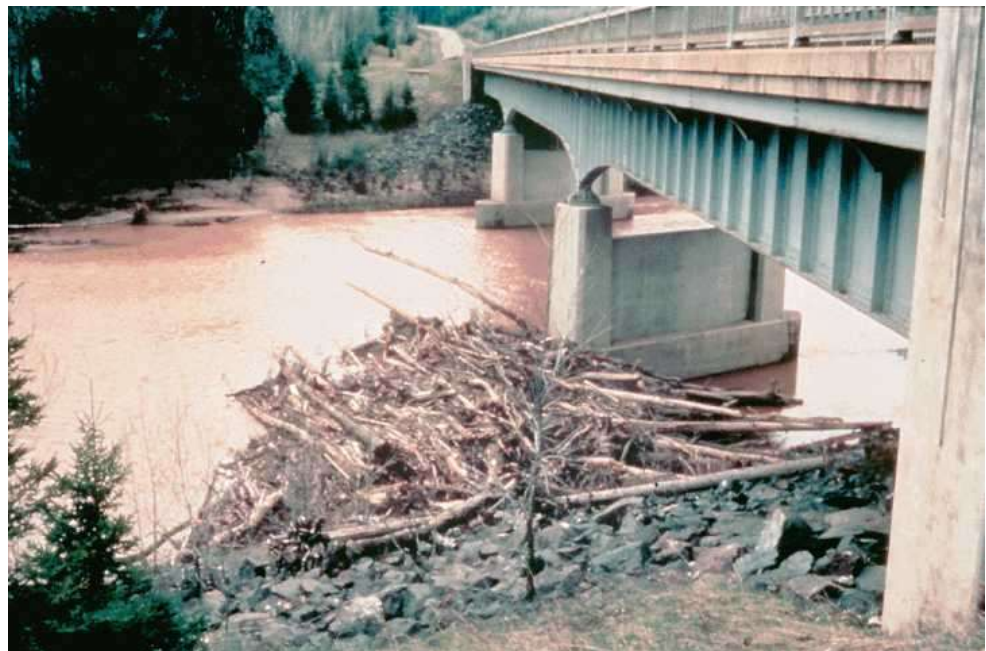
Figure 13.2.12 Debris Build-up in the Waterway
