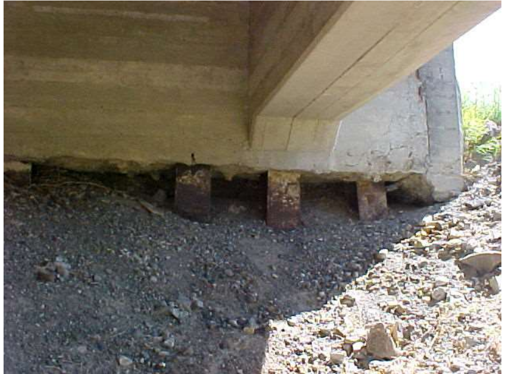
Figure 13.2.58 Exposed Piling Due to Scour
