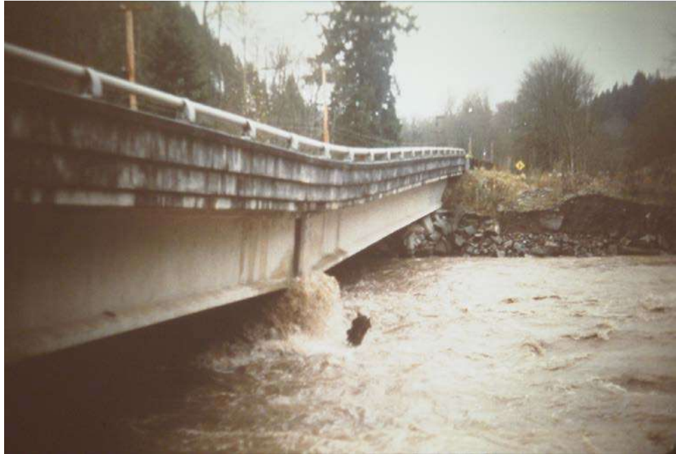
Figure 13.3.12 Movement of a Substructure Unit
