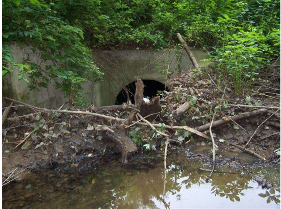
Figure 14.1.28 Debris and Sediment Buildup
