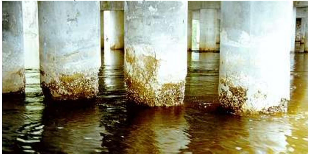
Figure 13.2.35 Pile Bent Deterioration Normally Hidden Underwater
