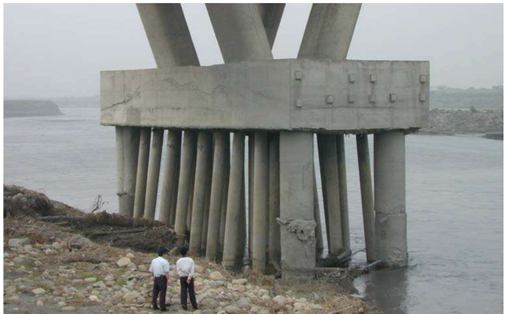
Figure 13.2.5 Close-up of General Scour of a Pier
