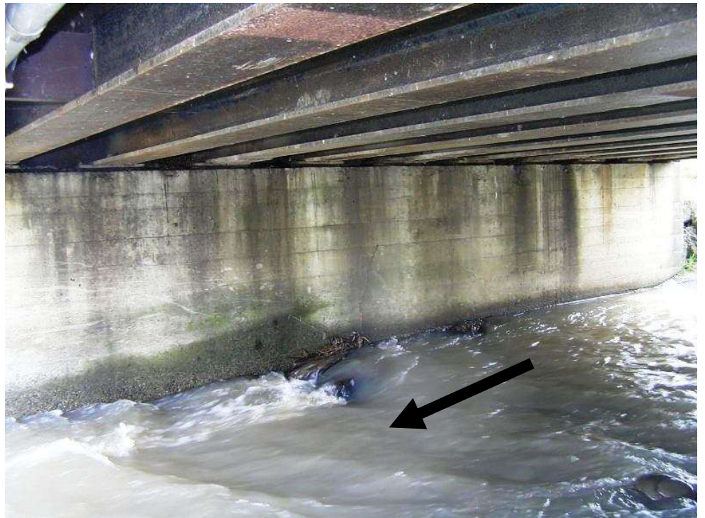
Figure 13.2.59 Accelerated Flow Due to Constricted Waterway
