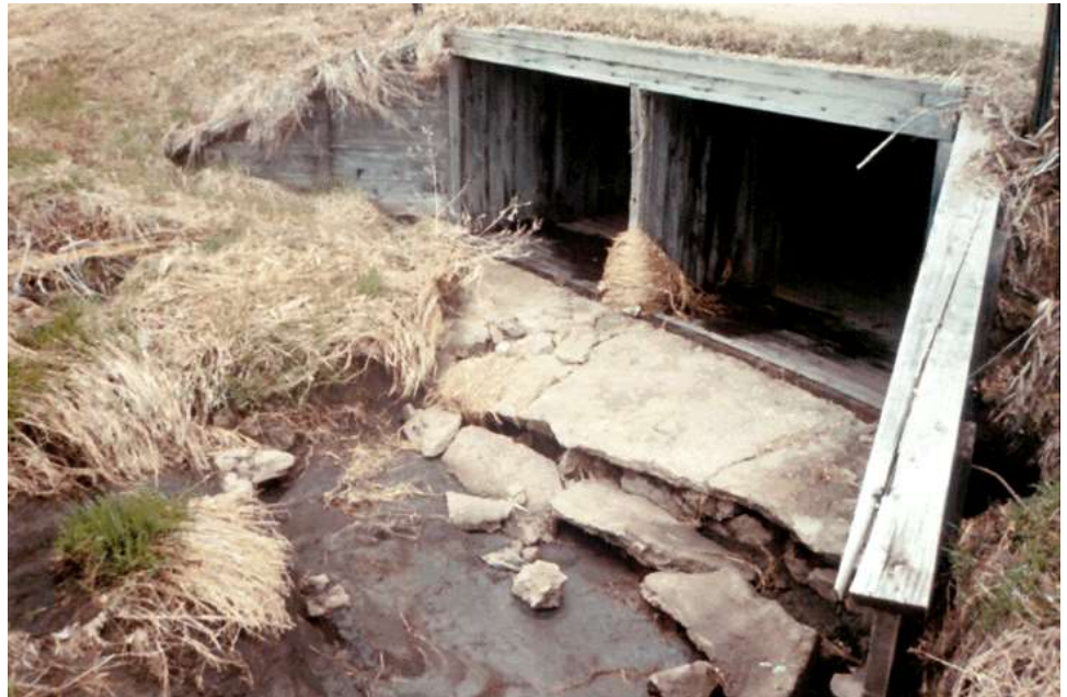
Figure 14.1.27 Scour and Undermining at Culvert Inlet
