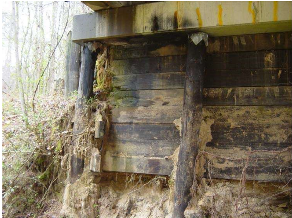
Figure 13.2.50 Scour at a Pile Abutment
