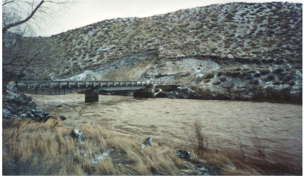
Figure 13.3.20 Severe Flood-Induced Abutment Scour
