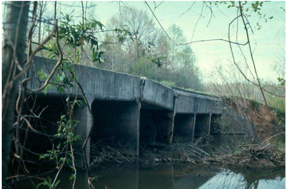
Figure 13.2.57 Rotational Movement and Failure Due to Undermining
