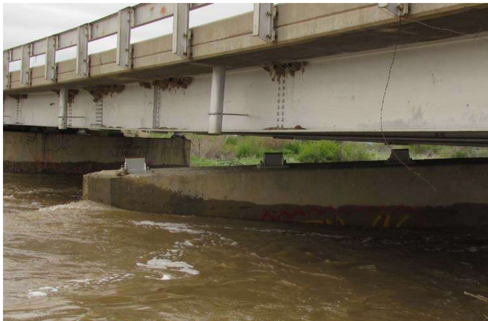
Figure 13.3.10 Flood Conditions: Pier Settlement.
