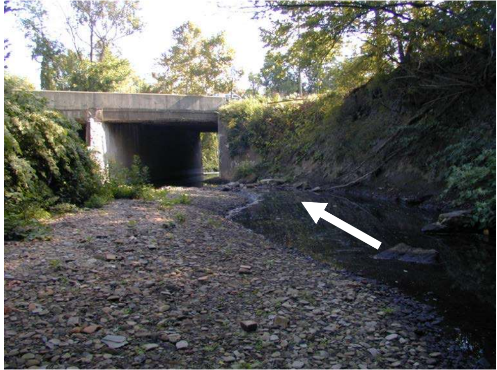
Figure 13.2.53 Typical Misaligned Waterway
