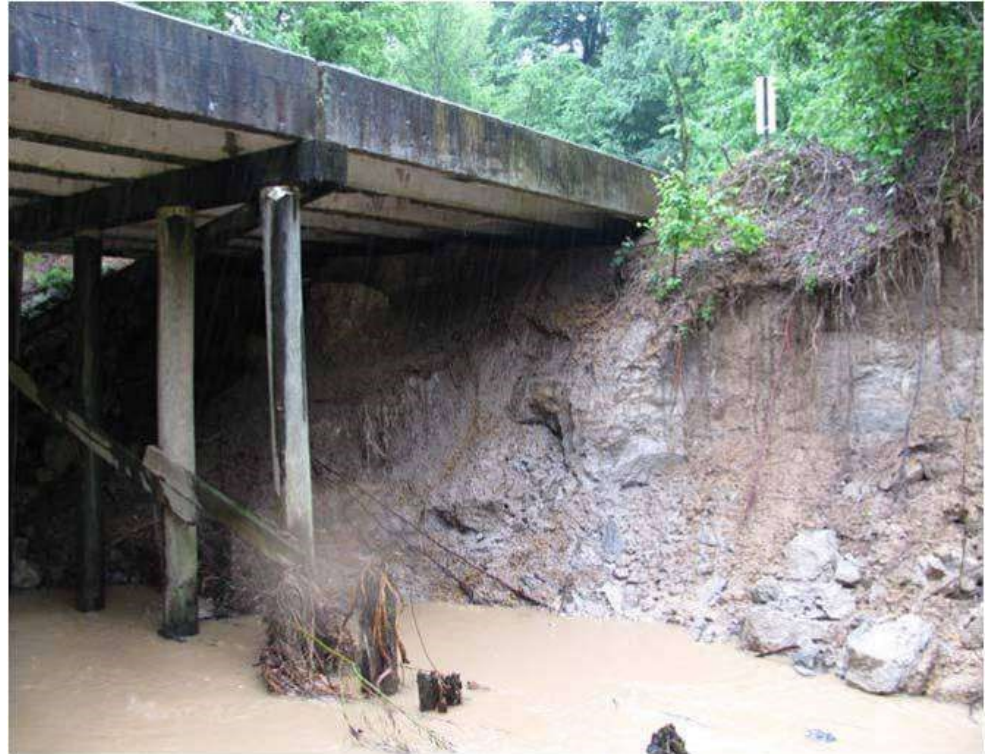
Figure 13.2.17 Lateral Stream Migration Endangering an Abutment
