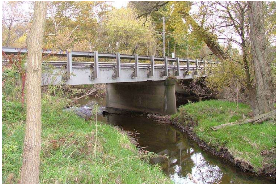
Figure 13.2.44 Sediment Accumulation Redirecting Streamflow
