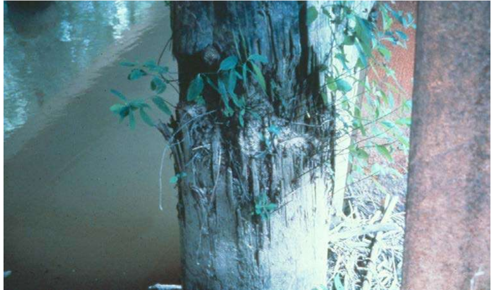
Figure 13.3.24 Deteriorated Timber Piling
