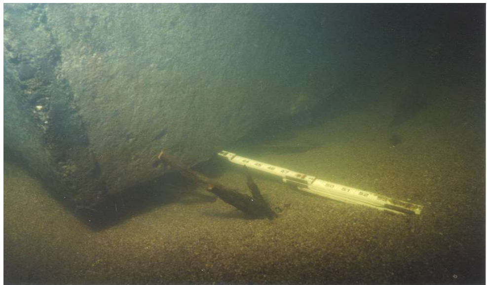
Figure 13.3.8 Local Scour; Causing Undermining of a Pier
